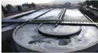
Akhisar Municipality Wastewater Treatment Plant
